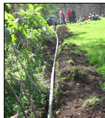
Pipes in place to carry water from the source storage tank to the community (July 2015)
