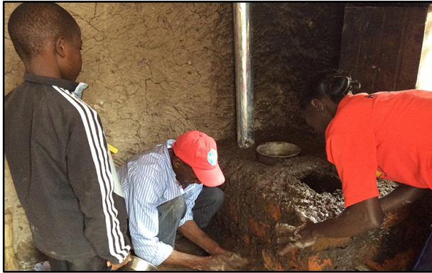
Friends of Londiani trains community health workers to install smokeless stoves using locally available material
